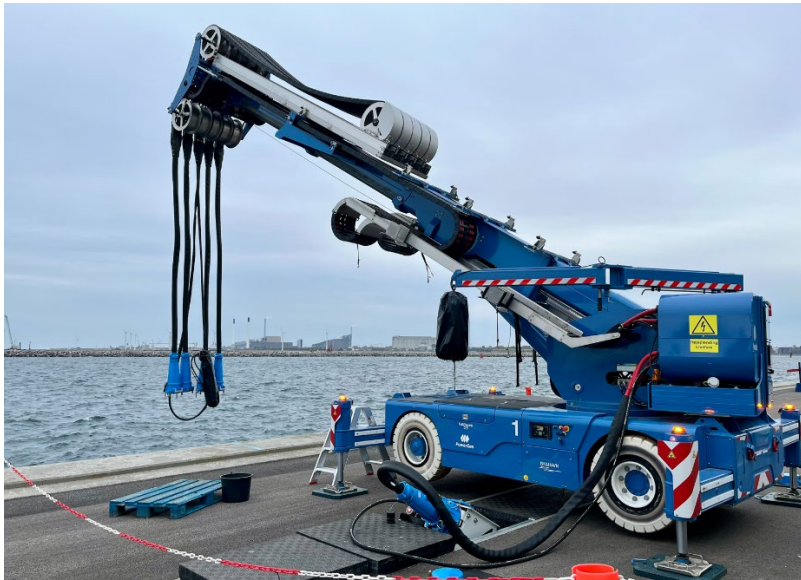
Figure 8-9 Example of quay-side electrical charging infrastructure at Copenhagen Port
