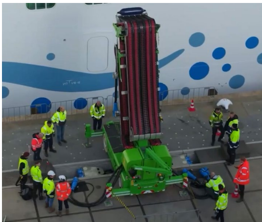
Figure 8-7 Cable management system connected to trenched shore-side sockets
