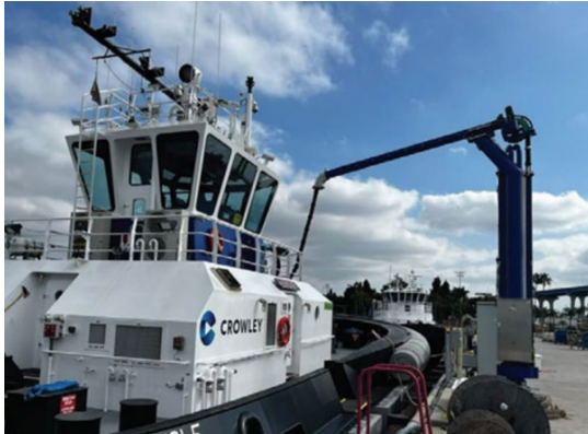
Figure 8-6 Dedicated berth-based charging arrangement for the electric tugboat eWolf, Port of San Diego
